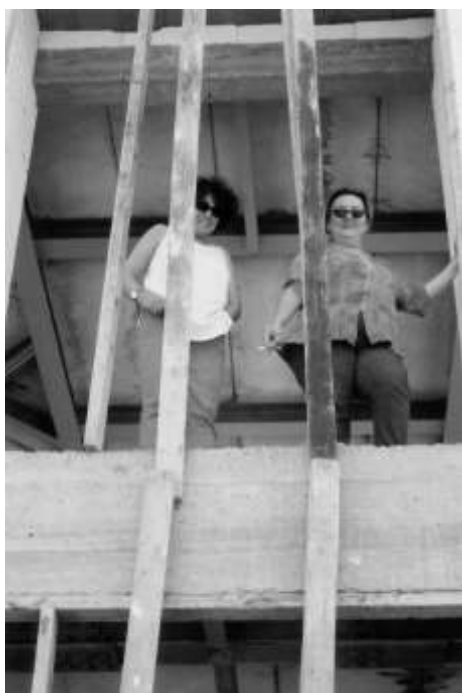
Women from KADAV overseeing the construction of a new women's centre © AI
